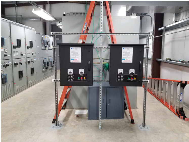
Final Installation, 2 of 6 High Resistance Grounding Devices
